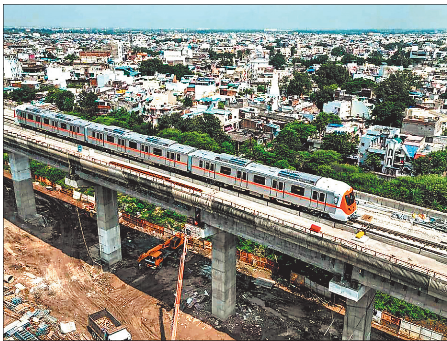
soon. During this period, two underground metro stations will be built. One metro station will be built near Nadra bus stand and the other near Bhopal railway station.
